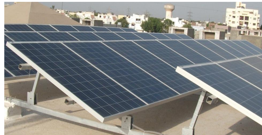
10 kW p roof-top solar PV system - Multi-crystalline
