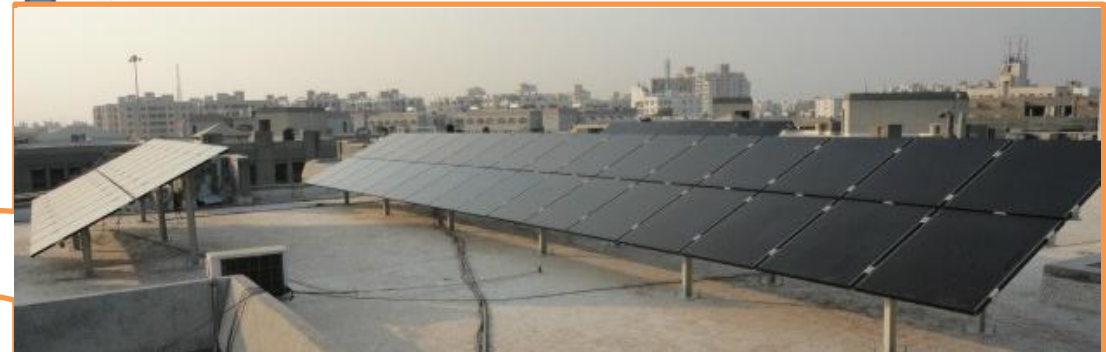
10 kW p roof-top solar PV system - Thin-film
